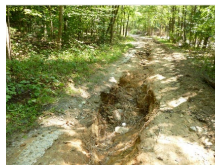
Figure 2: Eroded trails in Stream Valley parks. Credit: Fairfax County Park Authority.
